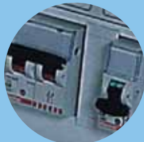
Main switch for the system
