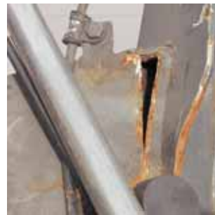
Coupling hinge damaged by the overhead wire
