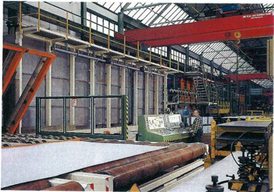
This vertical spray pickling plant has been rebuilt with solid metal segments in Nicrofer 3127 hMo - alloy 31 in highly stressed areas.
