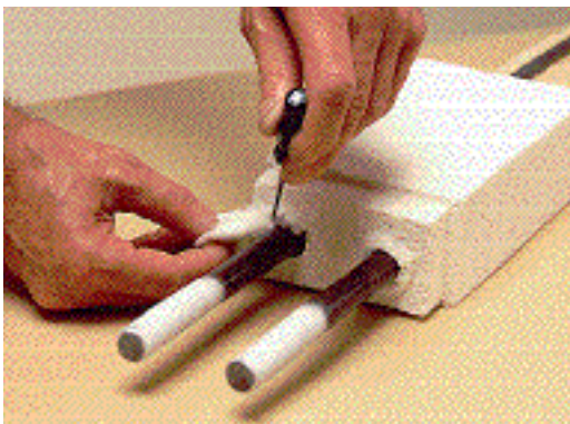
4. After packing heavy-duty ceramic fibre loosely into the recesses of the terminal holes
