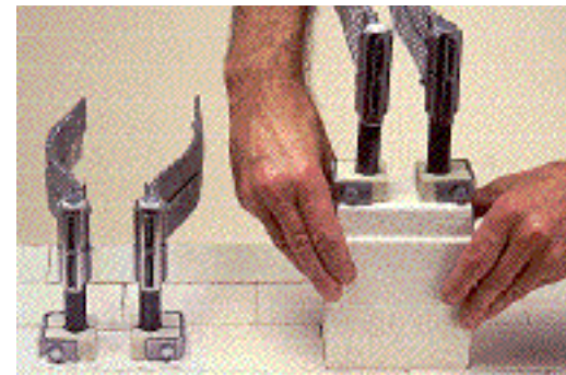
8. ...it is necessary to check the size of the corresponding holes in the roof.
